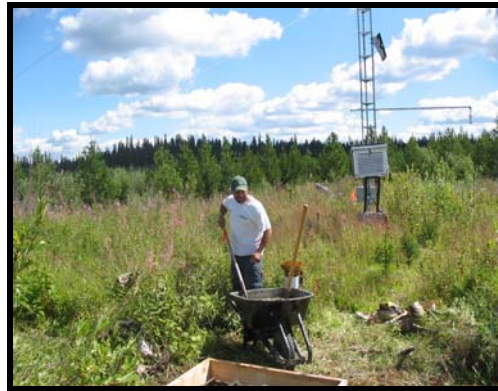
A new concrete foundation is prepared for the weather tower. ALRF staff refurbished and upgraded the weather station in October 2004 (Photo: M. Jull, Aug. 2004).
