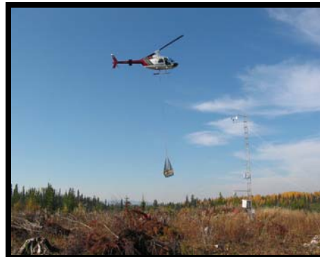
Helicopter slinging a rebar cage, for the new wind tower base, into the climate station site (October 2003). Work on the weather station will continue in 2004.
